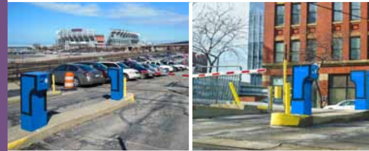
Parking System CrossPark USA, Cleveland
